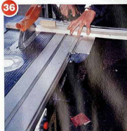
Cross-cut to length the stiles for all the four framed shelves. Do the same to two A and two B-type framed shelves, to create their final width
