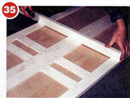
Cramp the two doors together and use them to measure the length of the stiles for all four framed shelves (marked A and B in the drawings)
